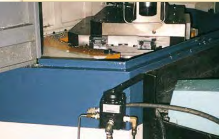
■ Enerpac VC-4 manual valves mounted to control hydraulic circuit on pallet fixture
