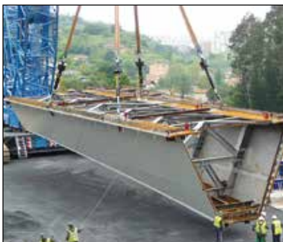
▼ Bridge segments are hoisted from the ground, being positioned with a 4-point SyncHoist system with fully monitorized cylinders.
